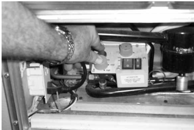
To run Refrigerator on Propane, Turn on Gas knob, Press and hold Grey knob and press Red igniter repeatedly until it lights.
